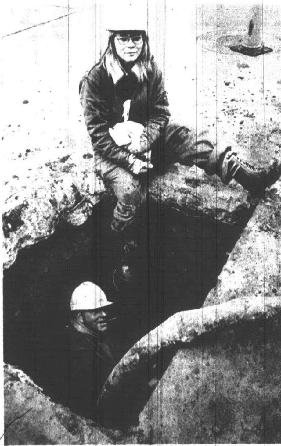
OUR ROVING photographer, Bob Woodring, caught these two Bell Telephone splicers working in a hole on Merriman Road. They are Ruth Bilyk of Dearborn Heights and Don Fowler of Plymouth. Ruth, incidentally, is the worker without the cigar.
