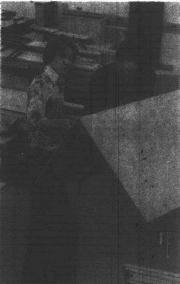
Rob Kuebler, junior, and Doug Hunter, senior, work on the roof for one of the miniature buildings in Safety Town. (Staff photo by Gary Caskey)
