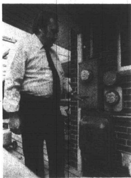
John Corrunker of Canton has two meters and a switching box for his windmill.
