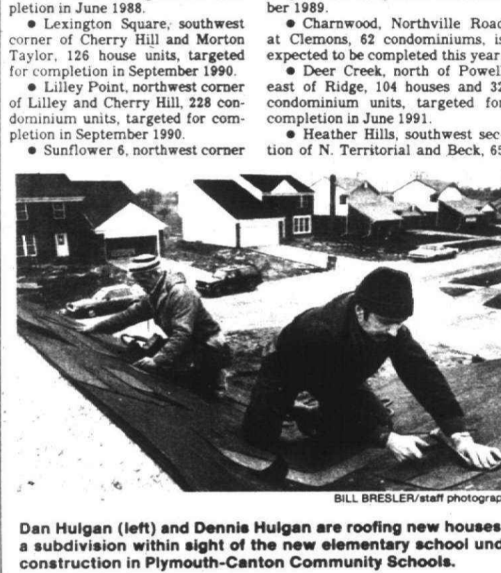
Dan Huigan (left) and Dennis Huigan are roofing new houses in a subdivision within sight of the new elementary school under construction in Plymouth-Canton Community Schools.
