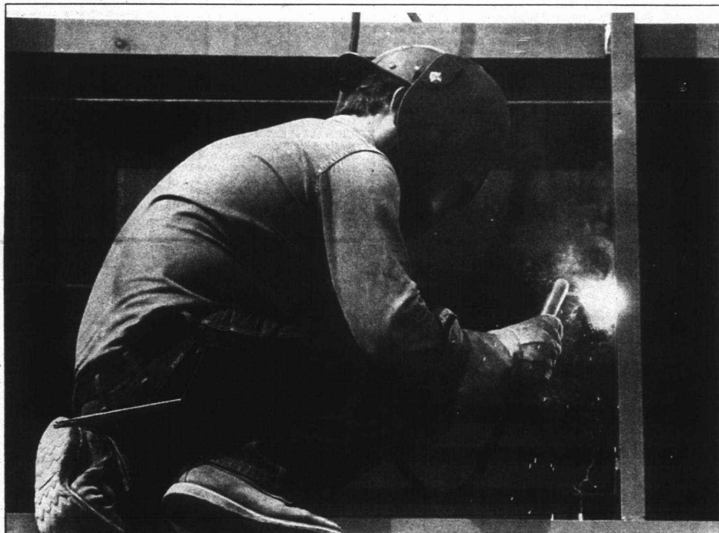
Eugene Hatmaker, arc welder, works on the addition to Oakwood Canton Health Center last week.
