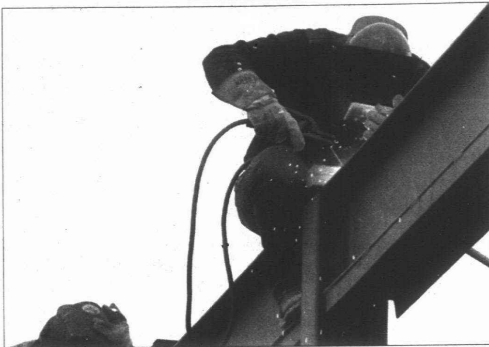
Postal progress: The only thing slowing new construction in Canton is likely to be the onset of winter weather. Pictured is a worker doing some welding at the post office on Canton Center, north of Cherry Hill.
