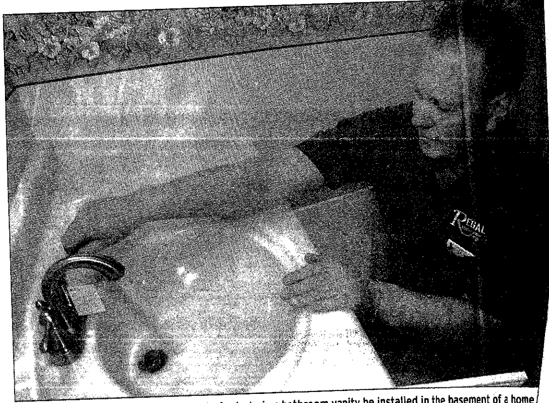
Tom Adamusik of Regal Construction checks for leaks in a bathroom vanity he installed in the basement of a home in Belleville.
