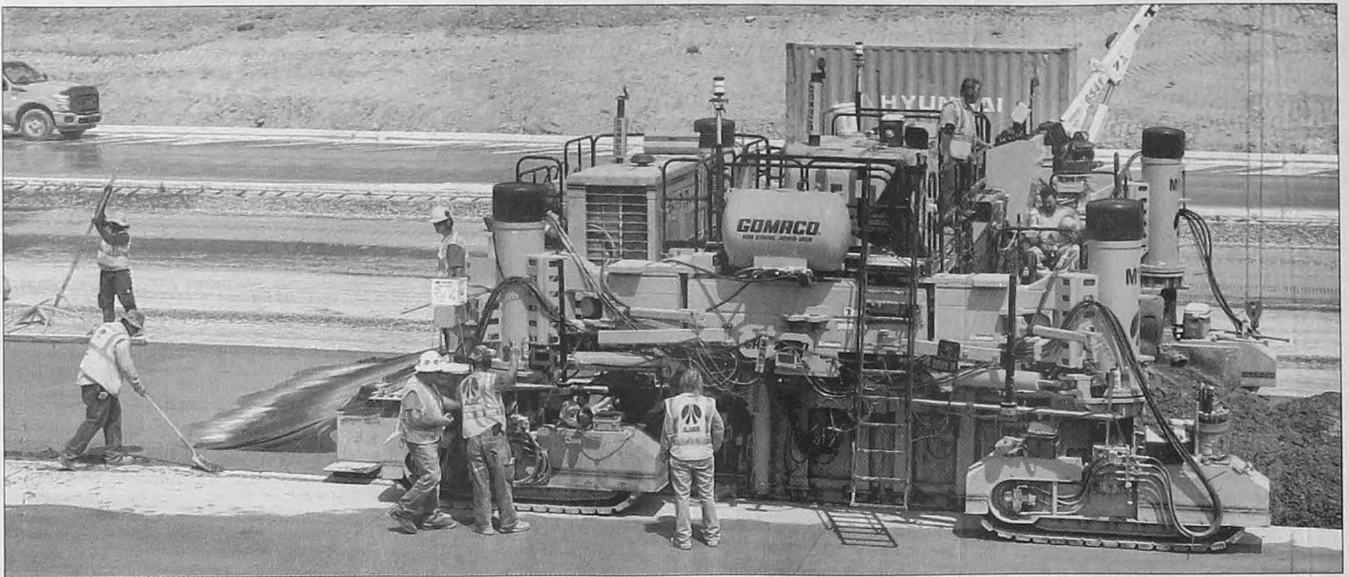
Miles of concrete are laid by machines like this. Mixed concrete is dumped in the path of the machine, which spreads and finishes the mix. PHOTOS BY BILL BRESLER | STAFF PHOTOGRAPHER
