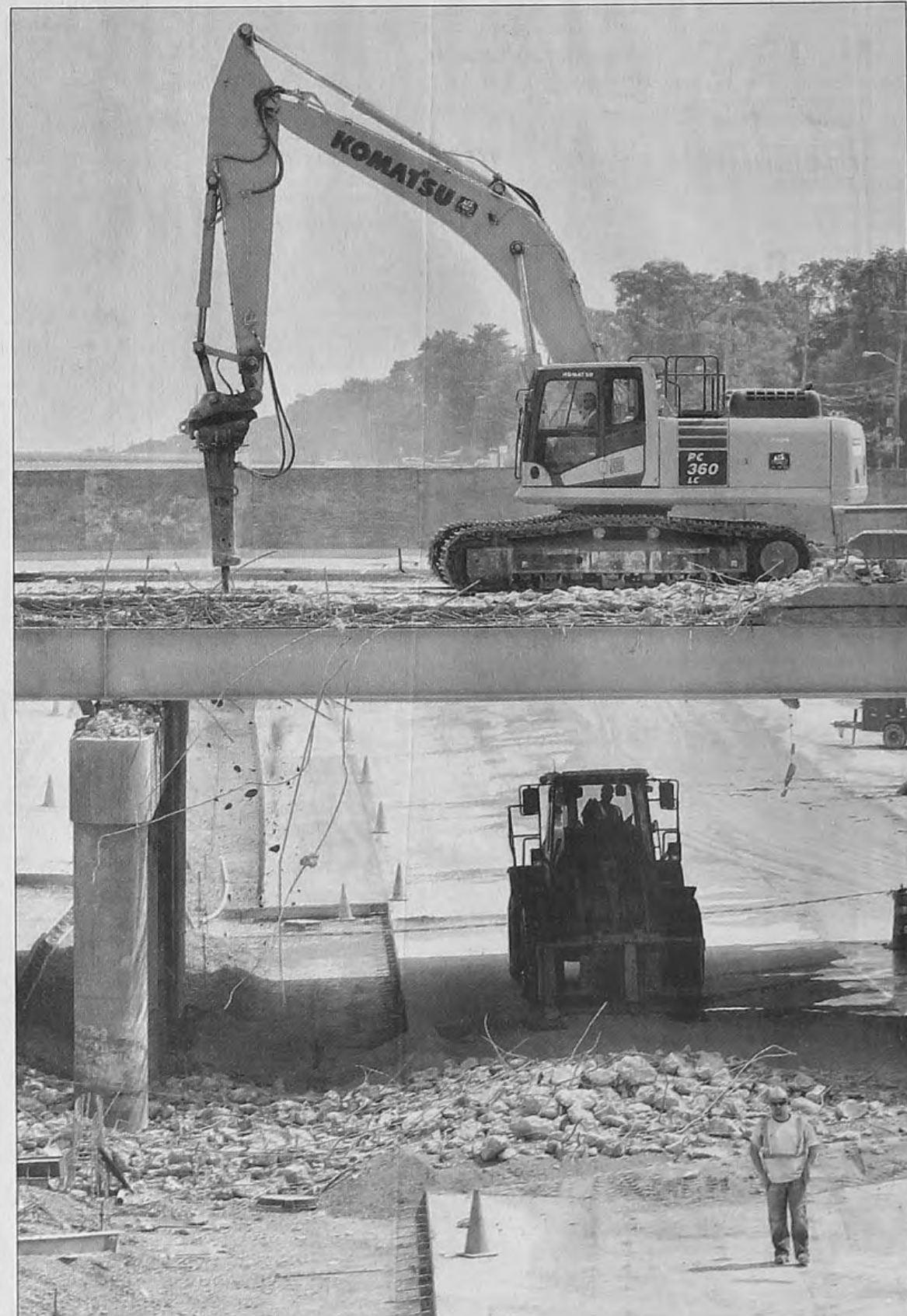
The road surface and side walls of the Beech Daly bridge are demolished, then rebuilt.
