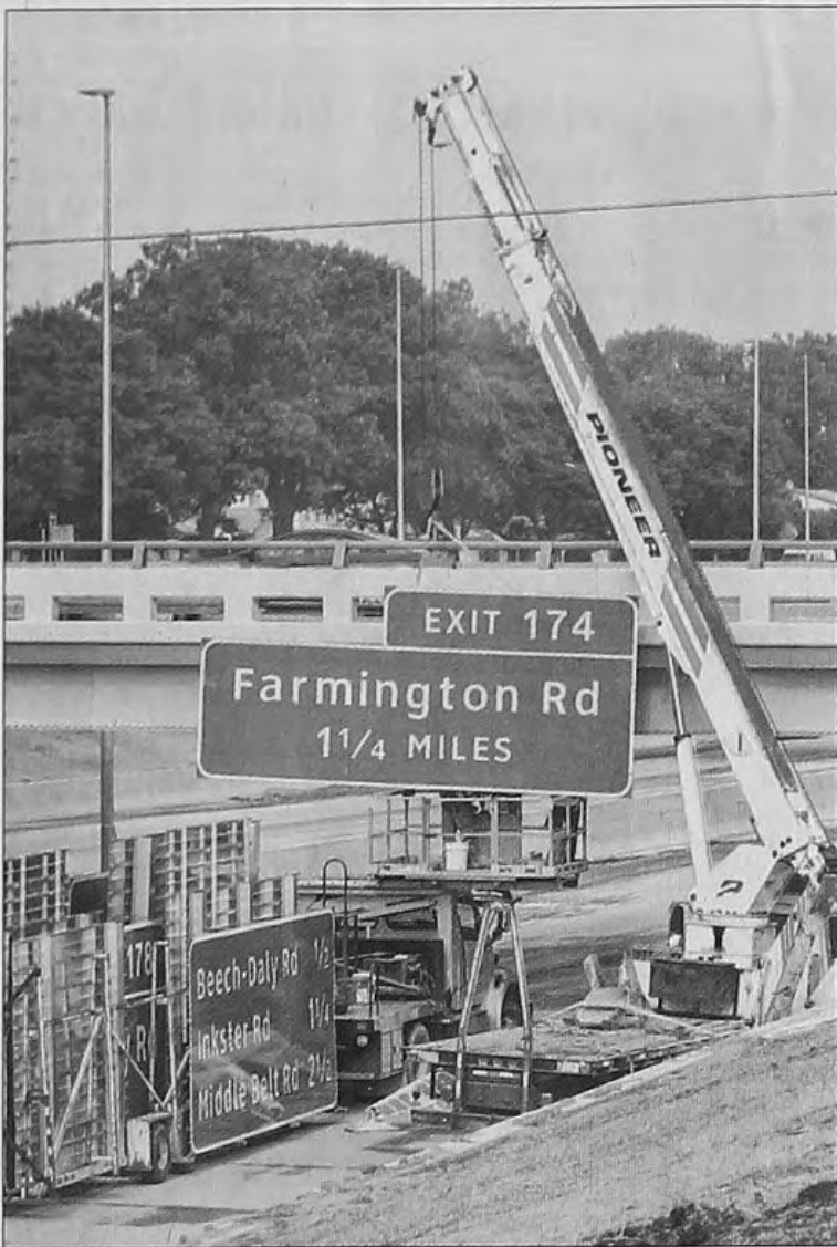
Workers mount new signs on the eastbound lanes of I-96 at Levan Road. Crews continue reconstruction on the freeway, which will open no later than mid-October through Redford and Livonia. Michigan Department of Transportation officials say the freeway will open all at once and will not open in segments. The $148 million project has left drivers seeking an alternate route since it closed in early April. BILL BRESLER | STAFF PHOTOGRAPHER
