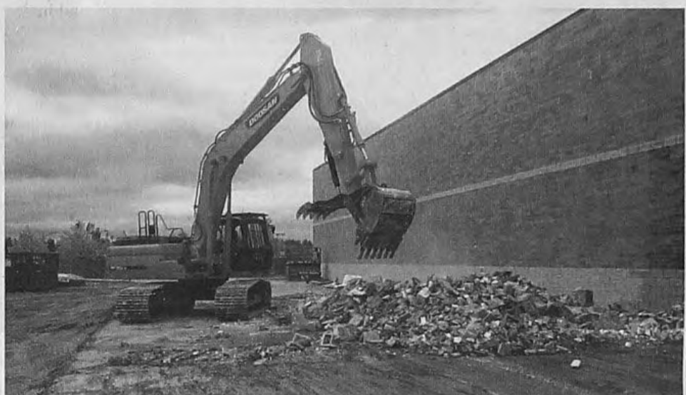
A crew from Detroit-based Blue Star Demolition begins the process of tearing down the former ABC Warehouse building on Ford Road to make room for expansion at IKEA.
