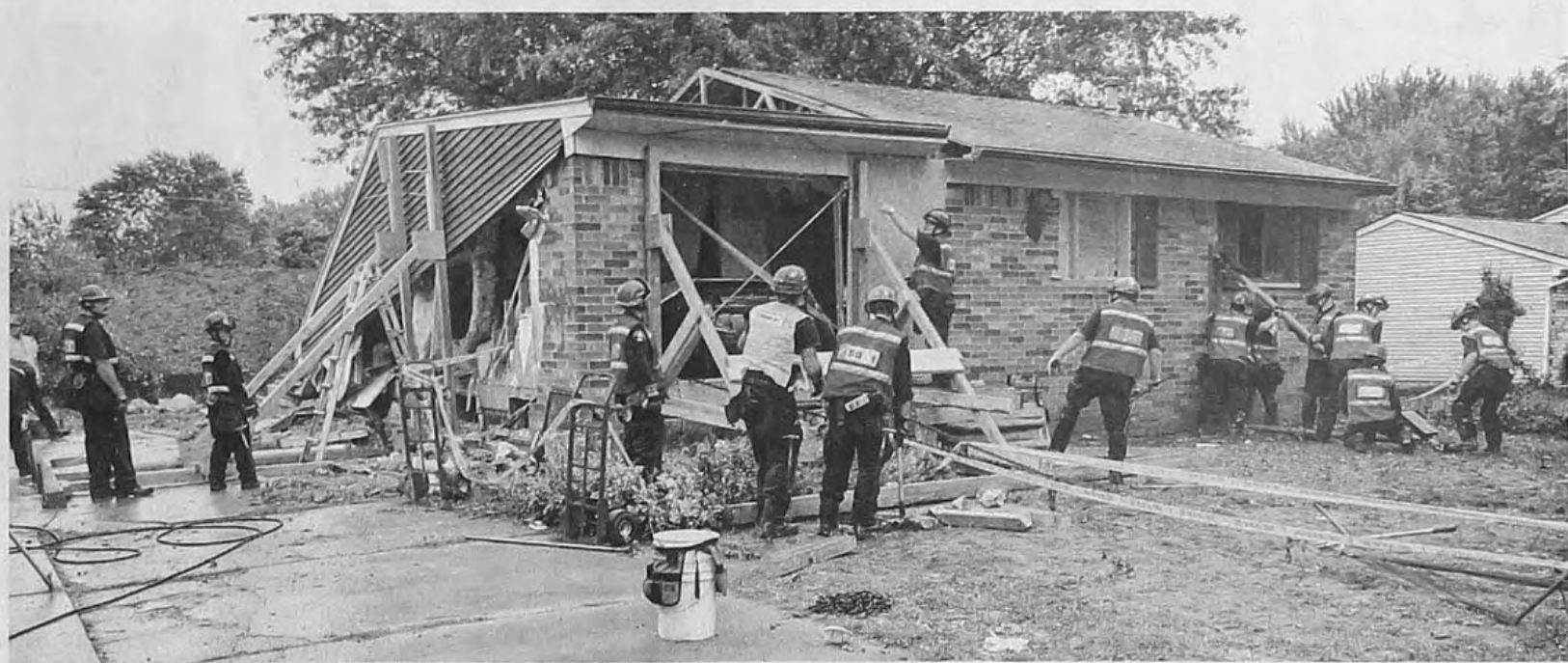
Although only the north side of the house has collapsed, the south side is supported to avoid a domino-effect collapse.
