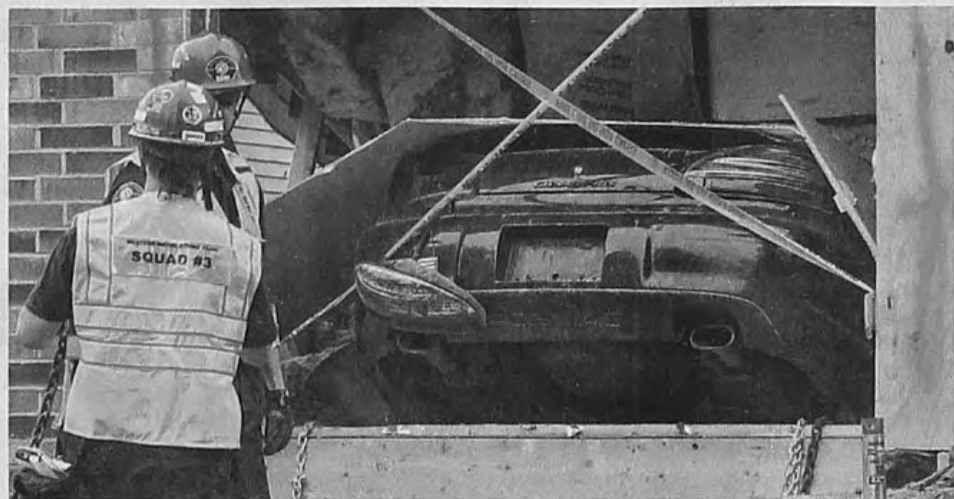
The scenario is that a car has smashed into a home, causing a partial collapse.
