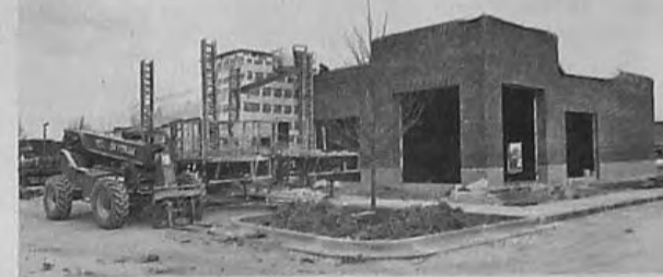
BILL BRESLER | STAFF PHOTOGRAPHER Bagger Dave's Burger Tavern is going up fast on Canton Center south of Ford.
