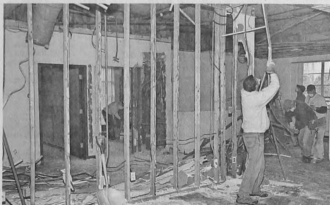
Crews work on the factory on the 14-acre site at Ridge and Cherry Hill roads.
