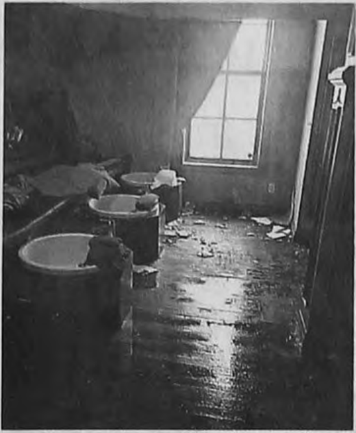
Water did extensive damage to the pedicure suite at Indigo Salon, Spa & Boutique.
