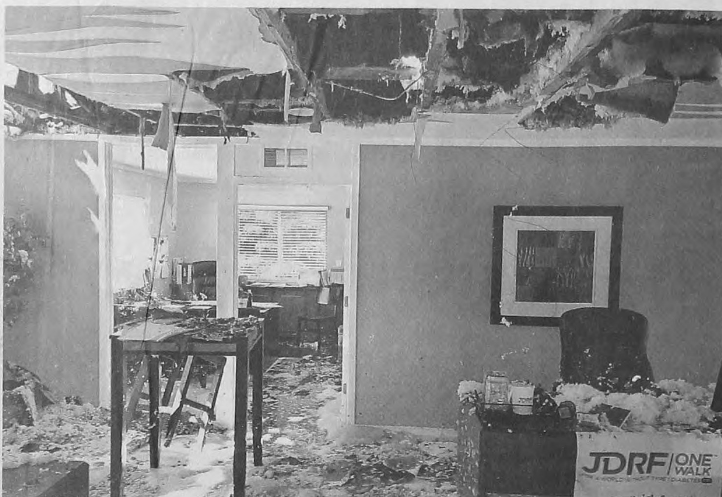
A fire left the interior of the Meadowood Townhomes clubhouse severely damaged.
