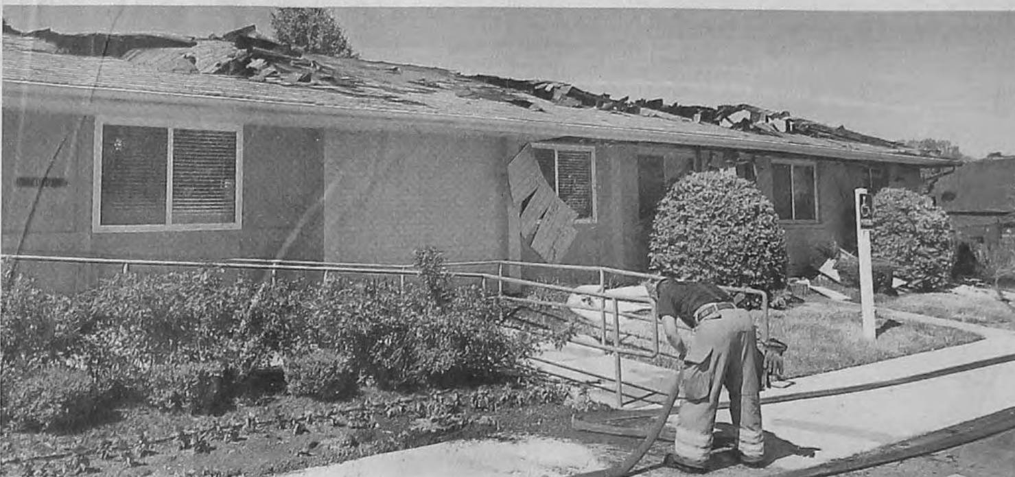
A fire at the Meadowood Townhomes clubhouse caused an estimated $150,000 in damage.
