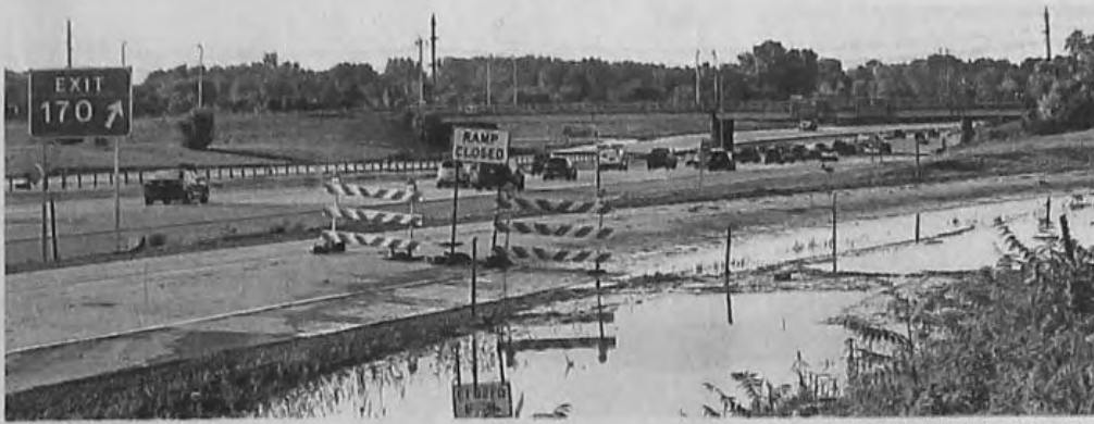
The ramp to Six Mile from southbound I-275 Wednesday morning. It was closed after flooding overtook the ramp for about 24 hours. The ramp reopened Wednesday.
