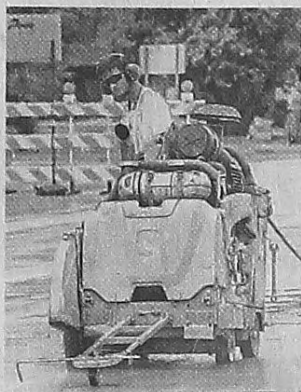
BILL BRESLER/HOMETOWNLIFE.COM Concrete cutting is underway. Removal of the old roadbed will begin soon.
