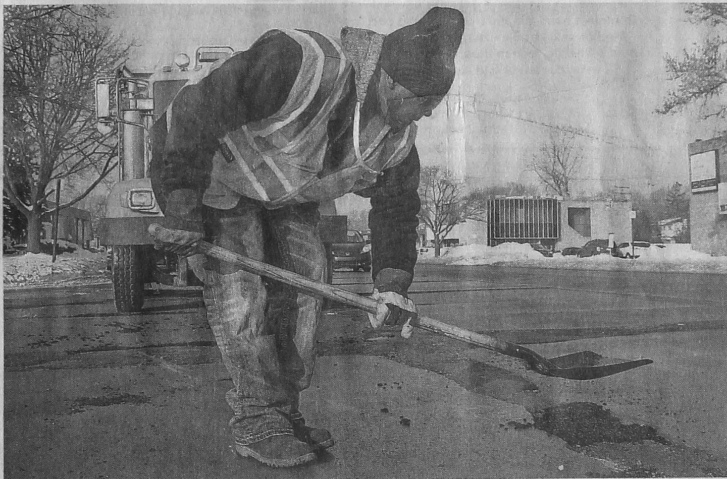
After filling the hole, Daimon Parker tamps down the patch with the back of the shovel blade. He knows the patch is temporary. Michigan's freeze-thaw cycle means that road crews never run out of work. BILL BRESLER | HOMETOWNLIFE.COM
