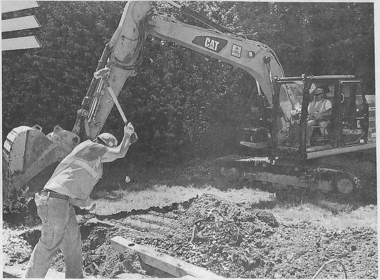
Tristan Stierley works the sledgehammer and Terry Benedict runs the excavator while removing a wall and several trees on the south side of the building. BRAD KADRICH | HOMETOWNLIFE.COM
