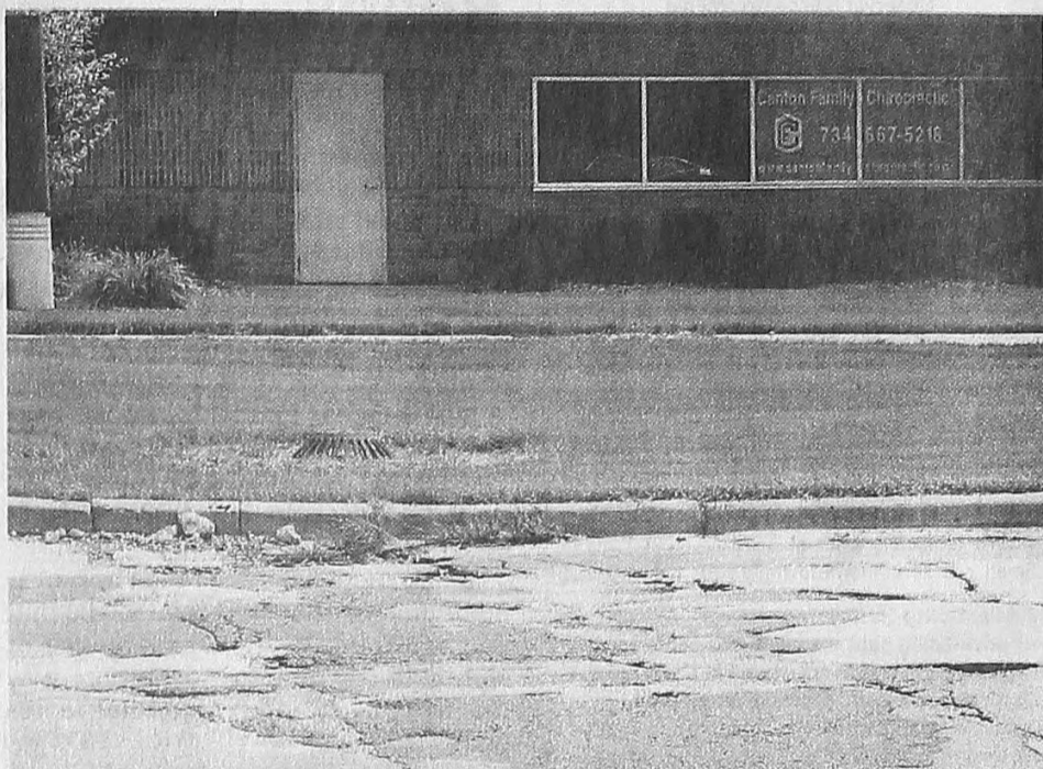
This rough patch of pavement on eastbound Cherry Hill Road will assuredly rank high on the getting-it-fixed priority list. ED WRIGHT | HOMETOWNLIFE.COM
