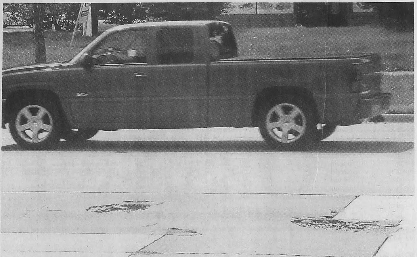
This pair of potholes on northbound Canton Center Road, just north of Hanford Road, is deep and dangerous. ED WRIGHT | HOMETOWNLIFE.COM
