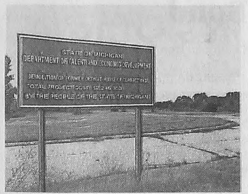
This former Detroit House of Corrections site, where buildings have been demolished, is pegged for redevelopment along the Michigan International Technology Center corridor. DARRELL CLEM | HOMETOWNLIFE.COM
