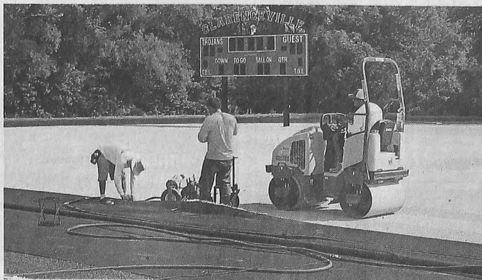
Workers are expected to install the new synthetic field turf field this week at Clarenceville's David B. McDowell Field at Tim Shaw Stadium. BRAD EMONS | HOMETOWNLIFE.COM
