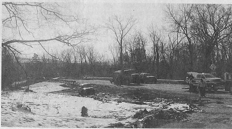
Members of the Wayne County Roads Commission remove barrels and barriers from the now-open Lilley Road bridge. ED WRIGHT/HOMETOWNLIFE.COM
