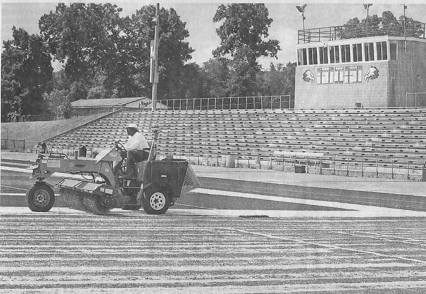
A renovation crew member spreads a cushioning layer of fine sand on Lakeland High's new artificial turf field July 14.
