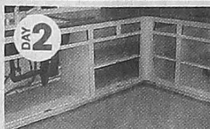
Your KURTIS craftsmen will cover all exposed surfaces with factory-finished materials
