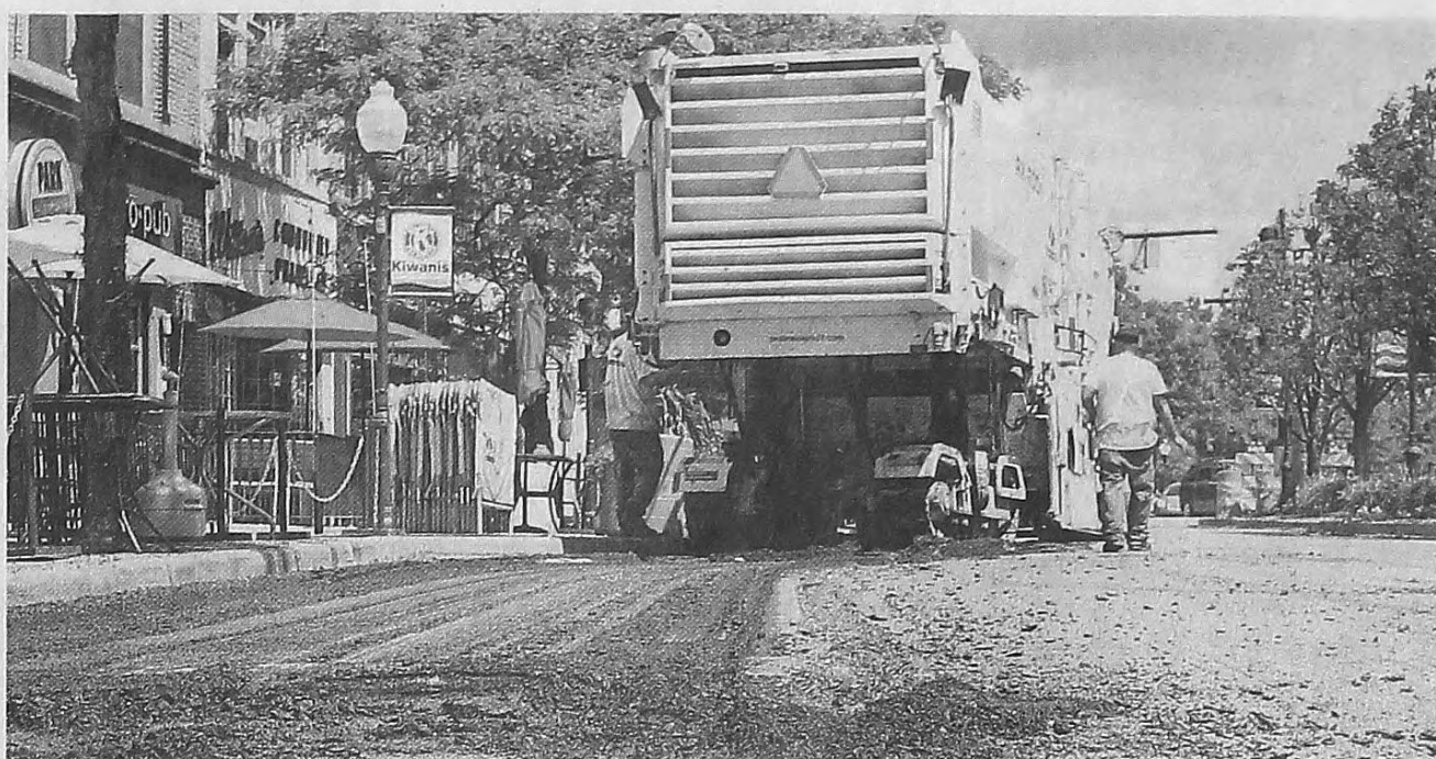
A road construction crew works on stripping a layer of the road surface on Main Street in Plymouth in July. JOHN HEIDER/HOMETOWNLIFE.COM
