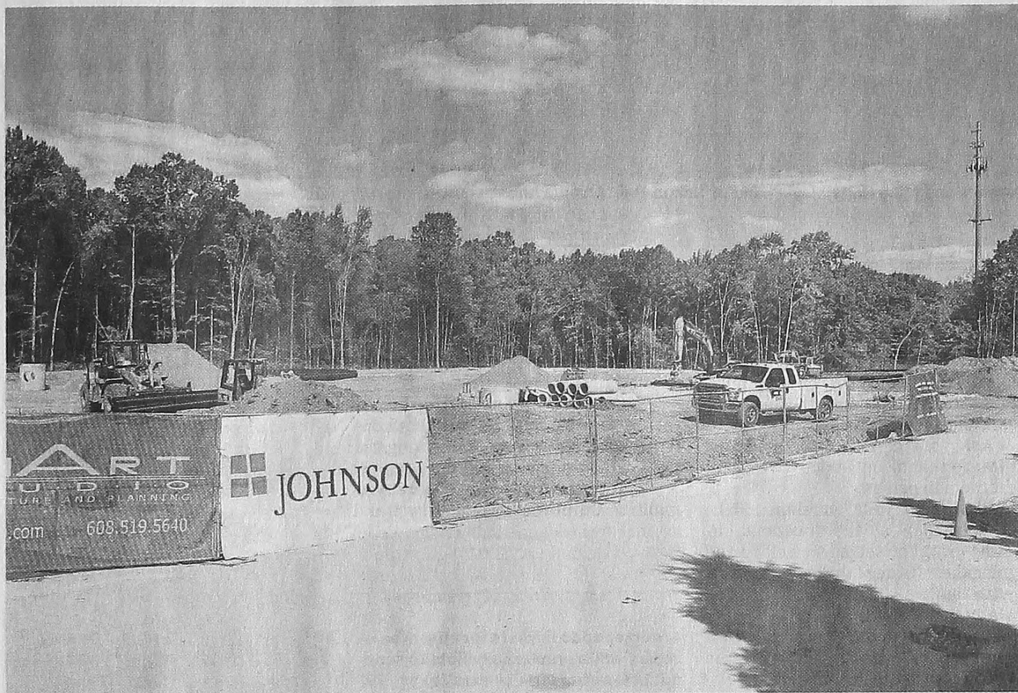
Construction of the VA medical center along Ford Road in Canton is still on schedule. JOHN HEIDER/HOMETOWNLIFE.COM
